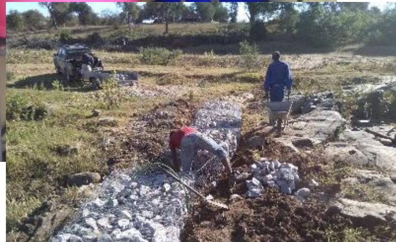
Protecting pipes and cables against floods and animals
